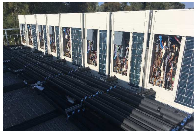
Mechanical condensers and associated pipework.
